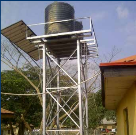
Rural Domestic Borehole
