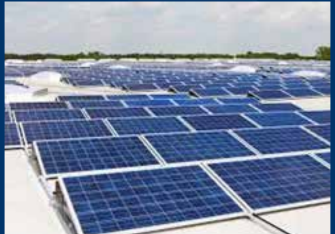
Commercial Rooftop Solar System
